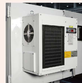
A/C for electrical cabinet
